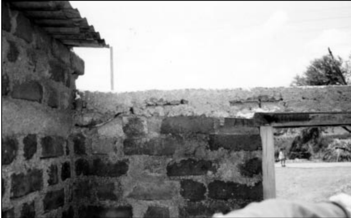
Figure 45 An example of poor construction of a concrete lintel band showing exposed rebar and the change in the level between the two walls.
